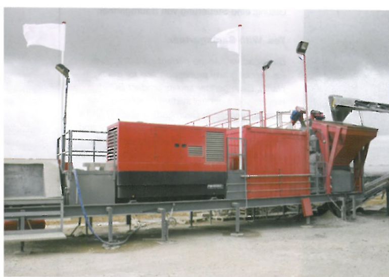
Photo shows the installation for high pressure cleaning of tools, the generating set, the cabin for operation monitoring and the inlet funnel above the mixer.
